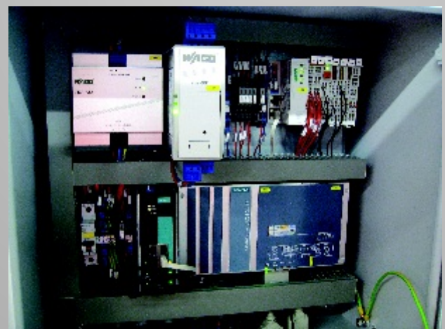
Electronics Cabinet with Embedded Computer and Peripheral Components
